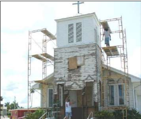
The Community Church got a facelift during restoration which took several months, beginning in June.
