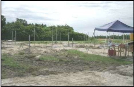
Progress is visible on the rebuilding of the hangars at ECity Airpark. They are scheduled for completion this winter.
