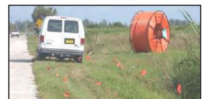
If you've been wondering what they're doing along the Trail, a new fiber optic cable is being installed for the School.
