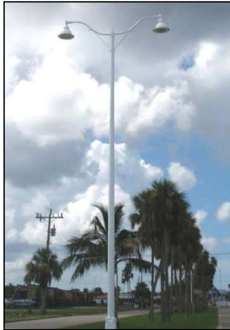
New street lights have been installed on Collier Avenue (CR-29) in the medians from the Post Office to City Hall. They will be turned on soon.
