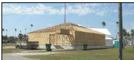
Work progressed on the new Louise Collier Jinkins Fellowship Hall behind Everglades Community Church. 6/10/11
