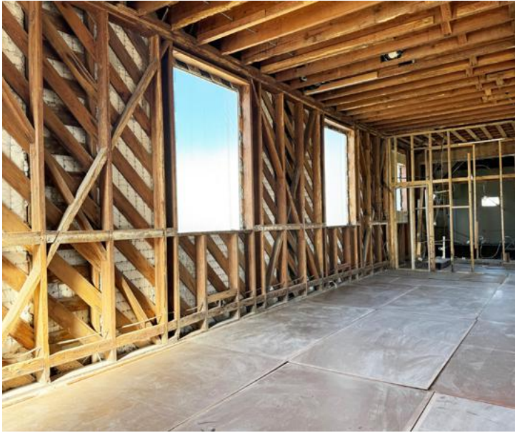
First floor restoration in progress – After removing the wainscoting (which will be cleaned up and reinstalled) and plastered walls, the structural integrity of the Bank of Everglades is clear. Built in 1927 with high-quality materials and expert craftsmanship, the building remains remarkably sound.
