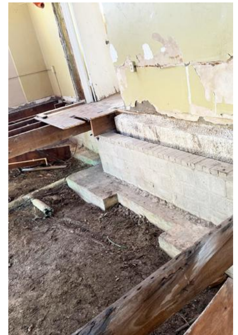
Exposing the vault's foundation – Removing the floor of the rear section of the building uncovered how an additional structural wall was poured next to the original foundation of the bank vault, a key feature of this historic building
