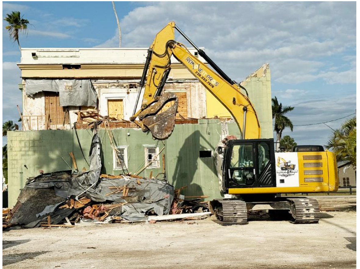
Removing the non-historic addition – This demolition clears the way for restoring the original Bank of Everglades building. The historic structure remains intact as part of the preservation effort.
